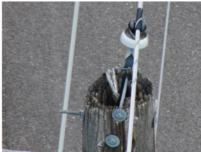
Figure 2: Example Drone Photo– Wood Pole with Decayed Top
